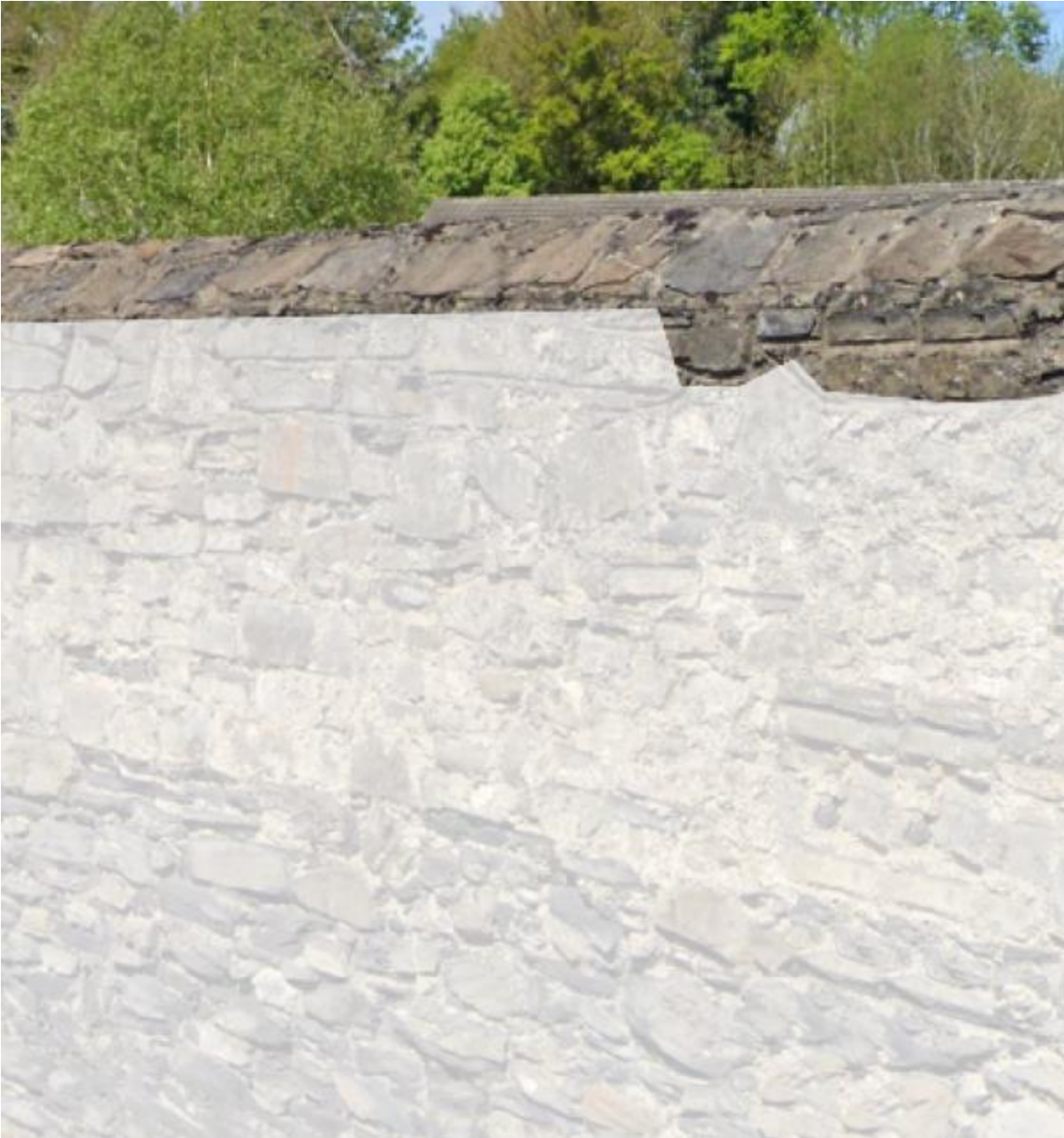
Figure 15 Upper section of wall which is consistent in profile along its entirety and shows a clear distinction in materiality between the lower sections suggesting modern addition
