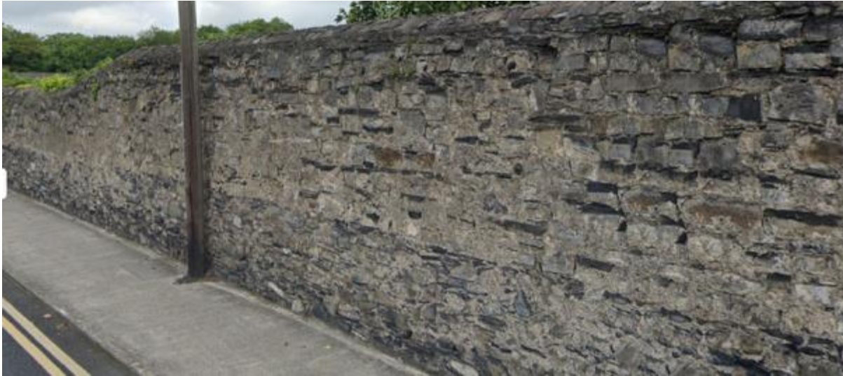
Figure 14 Clear distinction in stonework between upper and lower sections indicated by a datum which is consistent along the eastern and western sections of original wall.
