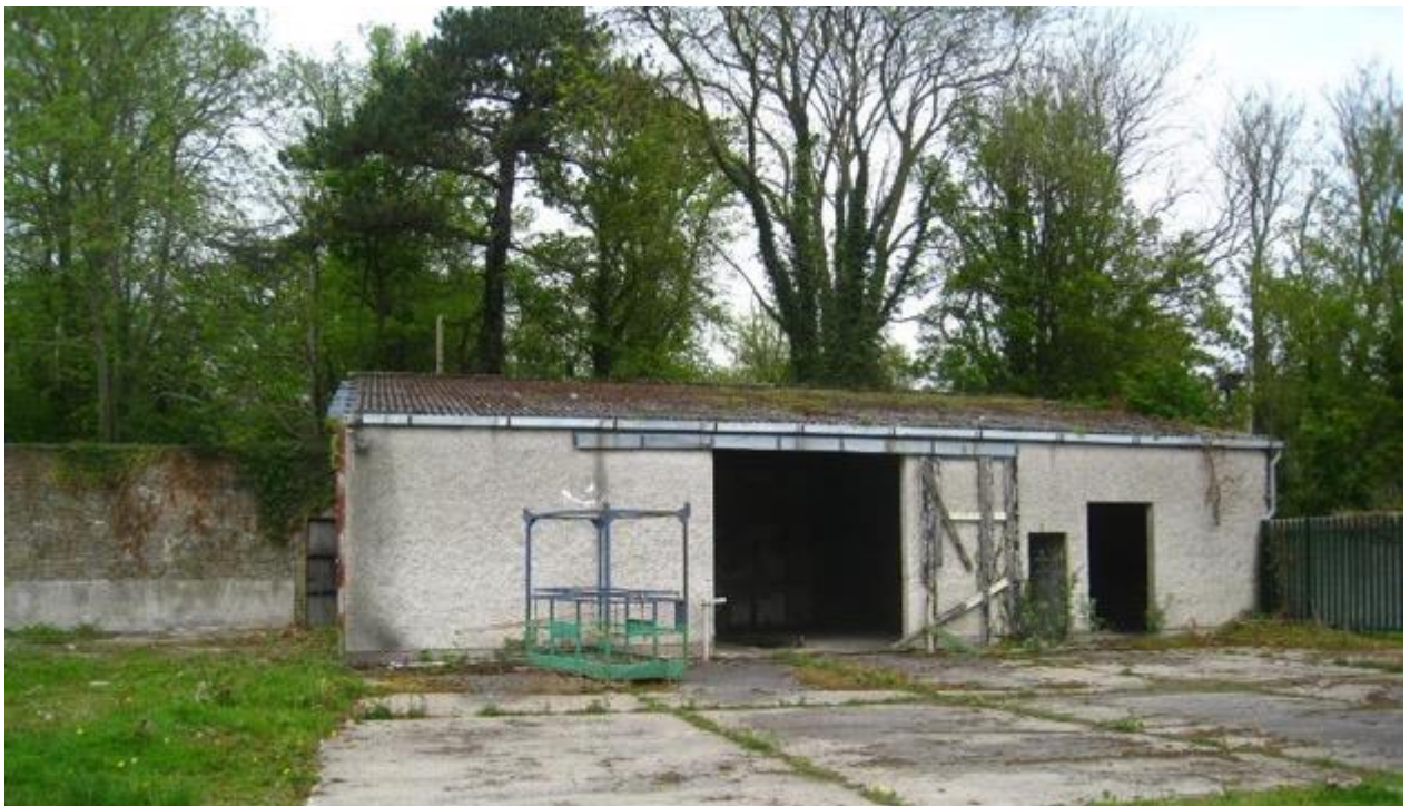
Fig.11: Non-historic ancillary building at the south of the north walled garden, proposed for demolition.
