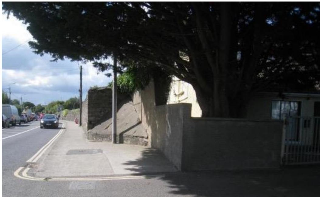
Fig.6: Non-historic section of entrance wall at the southeast of the site, proposed for demolition.
